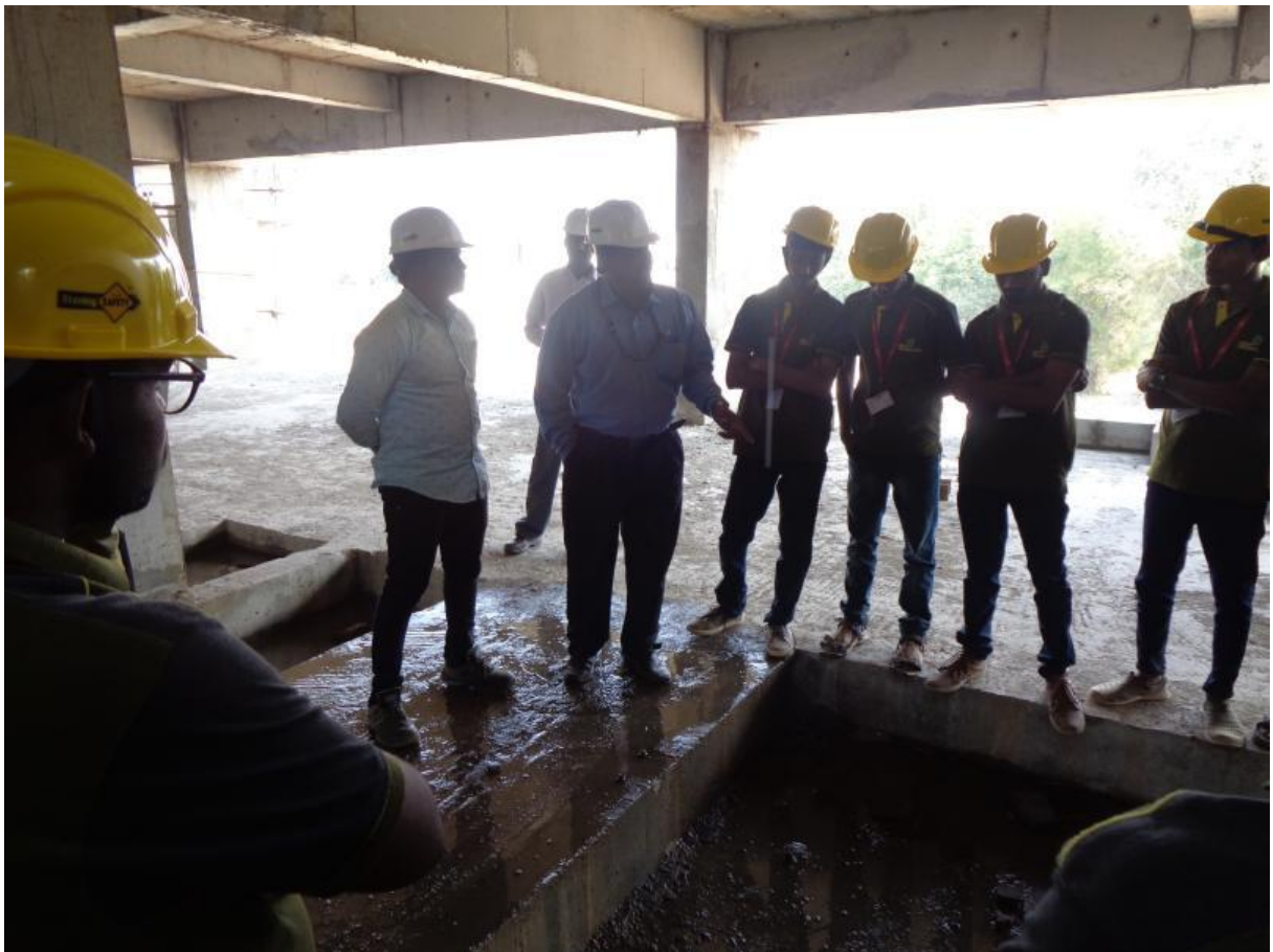
Dr. P. Ramesh and the site engineer explaining sunken slab
