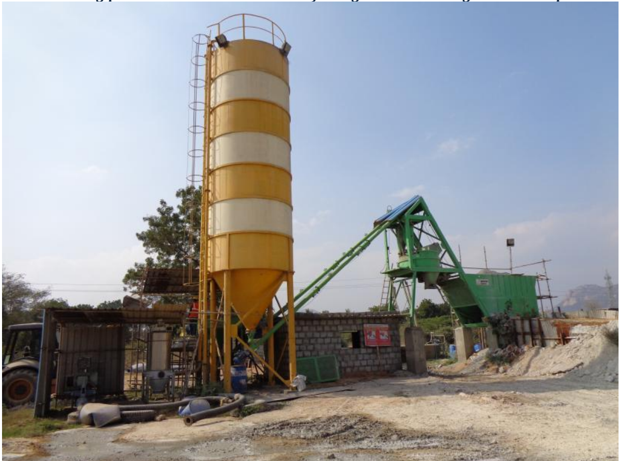
Batching plant at the construction site of college hostel building on SVEC campus
