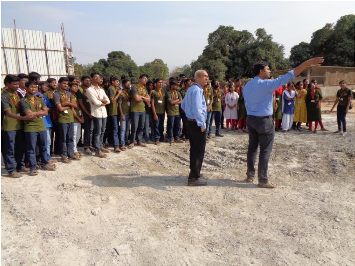
Dr. Hemadri Prasad Raju and Mr. M. Gokulnath explains the various components of batching plant at the construction site of college hostel building in SVEC campus
